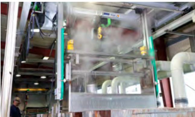
A special crane with height-reduced endcarriages and an individually adapted STD 50 dual chain hoist works in one of the largest burnishing plants in Germany.
