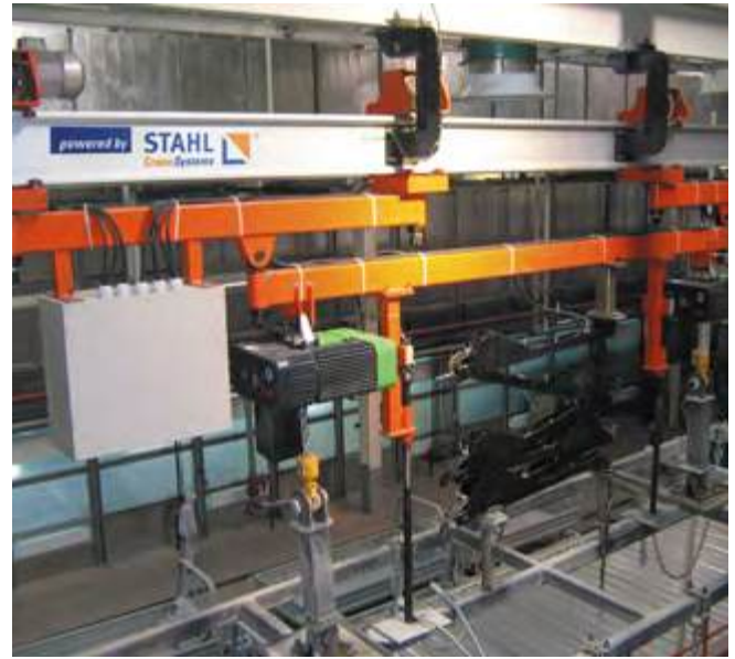
48 off-standard chain hoists operate in extremely high humidity in a coating plant for the motor industry in China.
