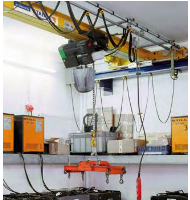
A chain hoist in short headroom trolley version is mounted on a single girder overhead travelling crane. It is used for transporting fork-lift truck batteries to the charging station.
