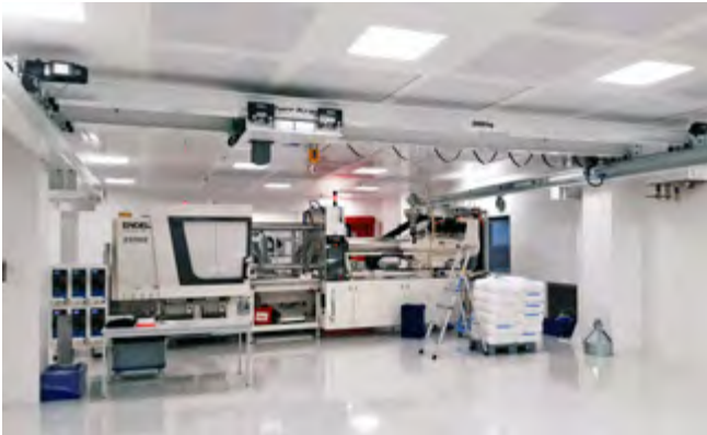
A special crane system with chain hoist is installed in a clean room facility. A drip pan under the hoist protects the production area below from possible abrasion particles.
