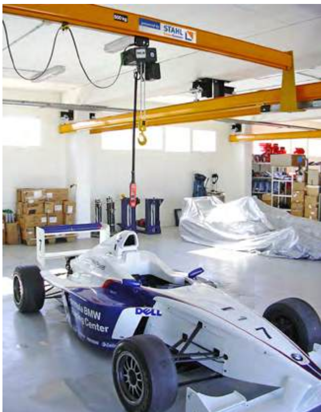
A light crane system with ST 05 chain hoists provides assistance in the repair, maintenance and servicing of racing cars.
